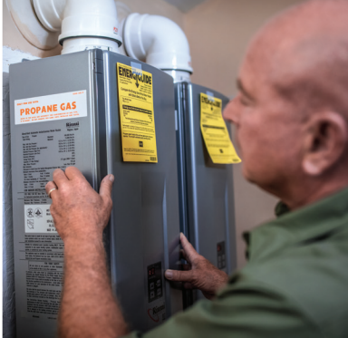
Propane Water Heater
